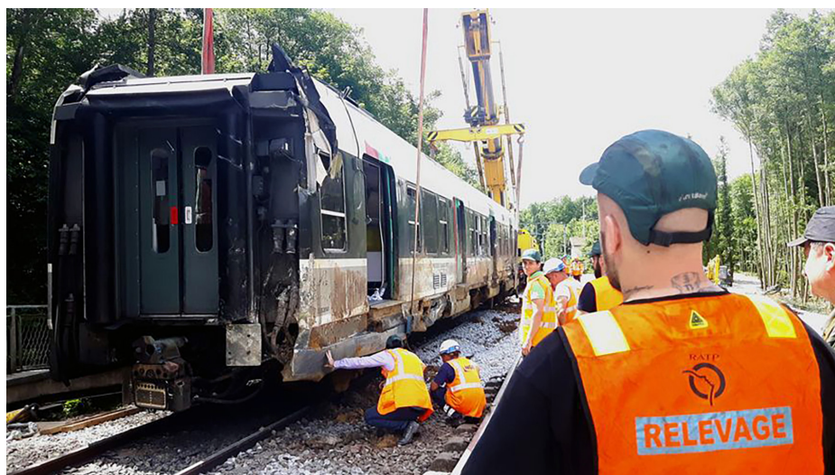
Re-railing of the RER B between Saint-Rémy-lès-Chevreuse et Gif-sur-Yvette. Source: Radio France - Emilie Defay
